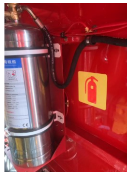
Fire suppression system
